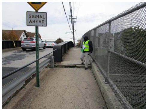
9. Uneven sidewalk on E. 32nd ramp - ADA noncompliance.
