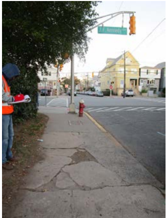
4. Severe sidewalk damage at West 11th and JFK
