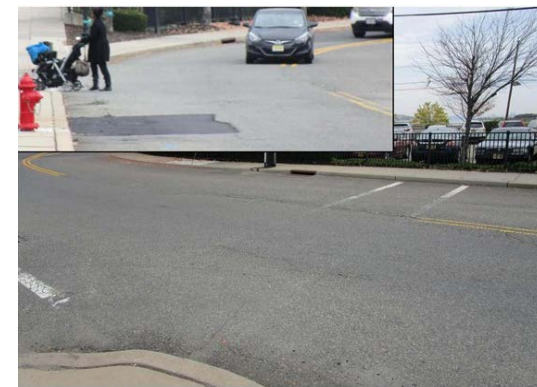
12. Missing curb cut / faded crosswalk on Prospect Avenue by 34th street station parking.
