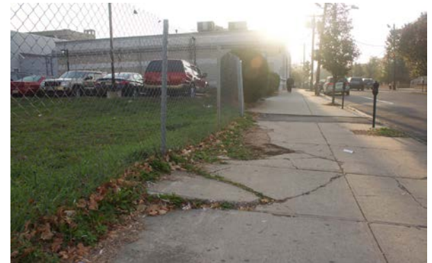
2. Severe sidewalk damage.
