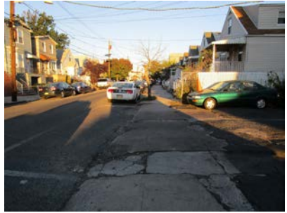
2. Severe sidewalk damage on West 12th and Broadway
