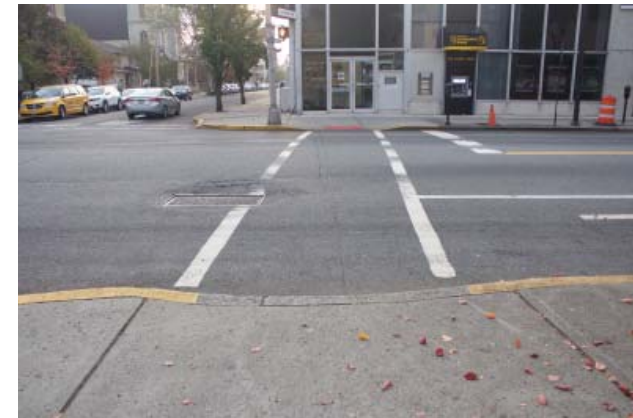
Missing truncated domes at West 26th Street & Broadway
