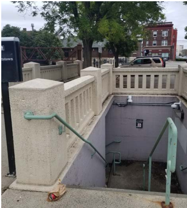
Figure 11: Lack of ADA Compliance for Station Entrances
