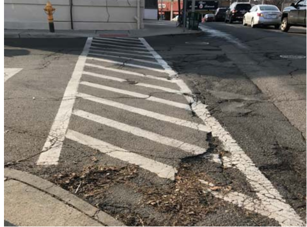
Figure 26: Cracked Pavement at Watsessing Station
