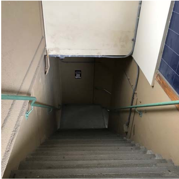
Figure 9: Poor Lighting in Station Stairwells
