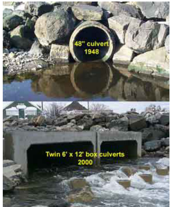
Fig.26. A culvert replacement project enacted to restore Little River Salt Marsh in North Hampton, NH. Credit: Natural Resource Conservation Service, USDA
