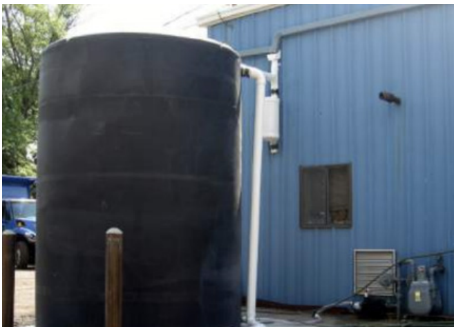
Fig.28. A cistern installed at a public works department in Clark, NJ. The rainwater is harvested from the rooftop of the building and used as part of a green car wash system.
