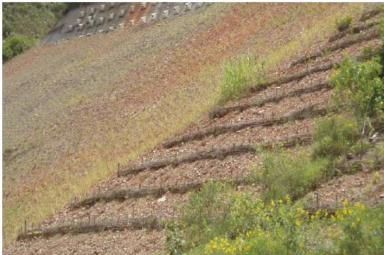
Figure 4. Newly installed live fascine on roadside (Image source: Western Transportation Institute by G. Keller, 2011)
